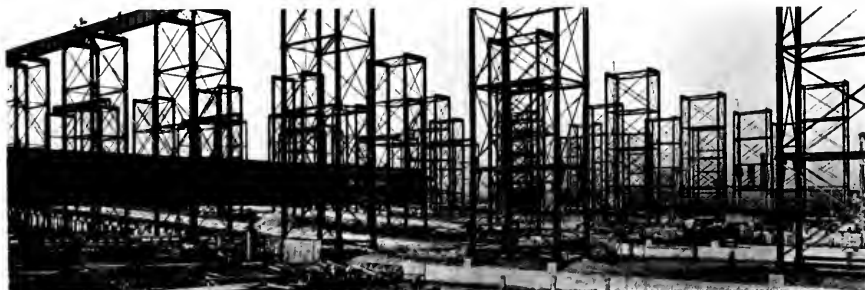
Steel work going up on the fine steel and concrete building berths of the Sun Shipbuilding Company.
